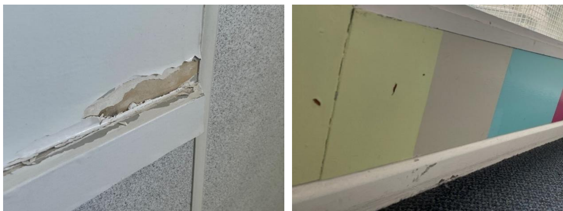
Photos of the bathroom and hallway that need repair
