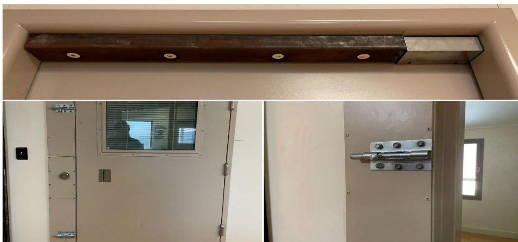
Secure room door with reinforcing bar and deadlocks on the outside of doors.
